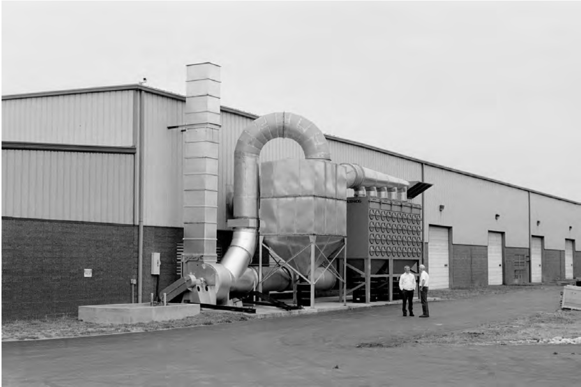
Figure 11.5. The furnace air filtration system.
