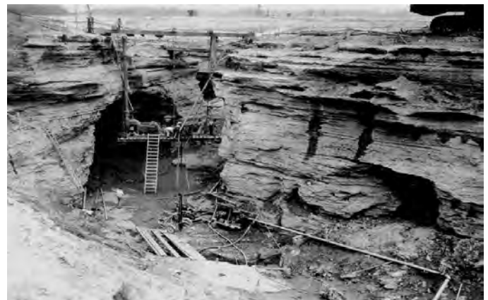
Cave and solution channels exposed in cutoff trench during excavations for Wolf Creek Dam, 1946. USACE engineers believe inadequate sealing of solution openings was responsible for the bypass leakage that plagued the dam ever since it was constructed. Source: Robinson (2015)., "Successful Foundation Preparations in Karst Bedrock of the Masonry Section of Wolf Creek Dam," in Proceedings of the 14th Sinkhole Conference, NCKRI Symposium 5, Carlsbad, NM, 2015.
